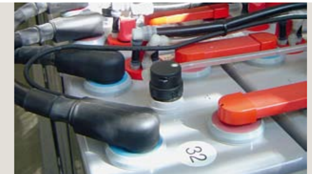
Storage technology New reserves for power grids
