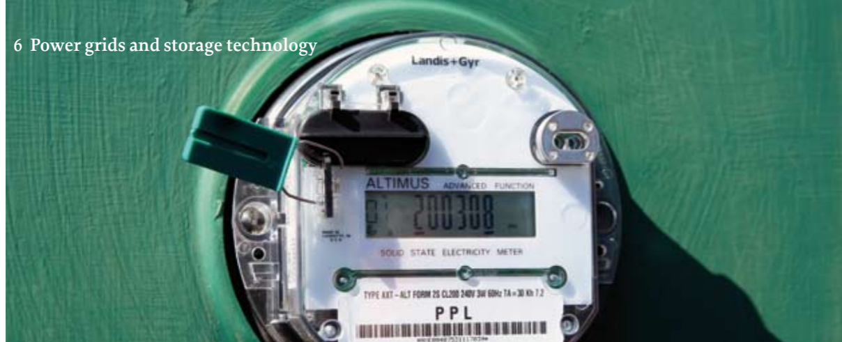
Electronic electricity meters provide the control centers with important information.
